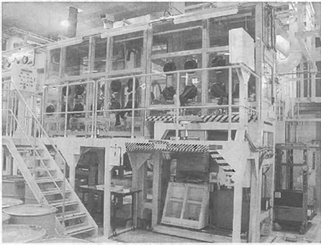
Fig.7 Filter Waste Processing Equipment
